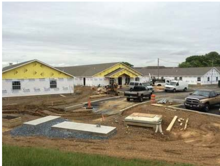
(Contributed Photo) Warfel Construction Co. is building Arden Courts, an Alzheimer's and memory care facility in Bethlehem Township.
